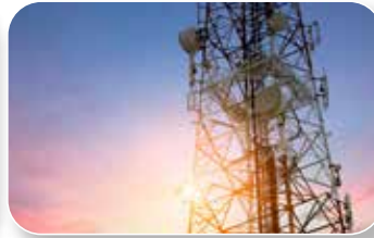
Radio Communication Equipment
